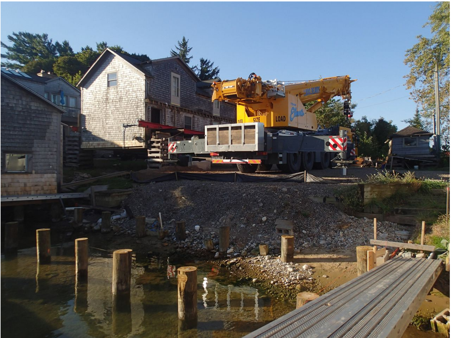
Fishtown's Otherside Shanty was lifted off its old foundation last year and recently returned to a higher, more solid perch. Photo provided by Amanda Holmes.
