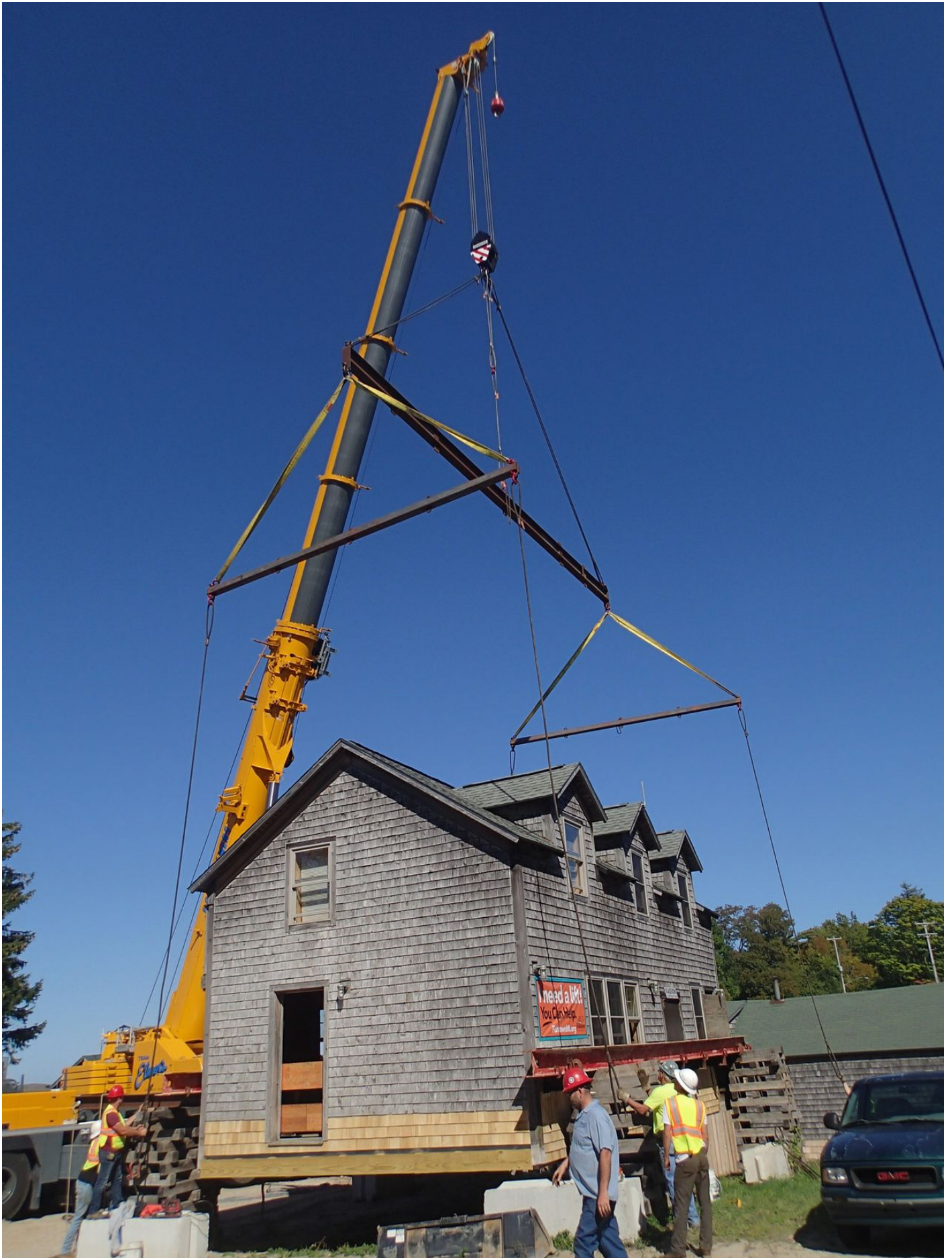
The Otherside Shanty had a date with a big crane to get it back in place. Photo provided by Amanda Holmes.
