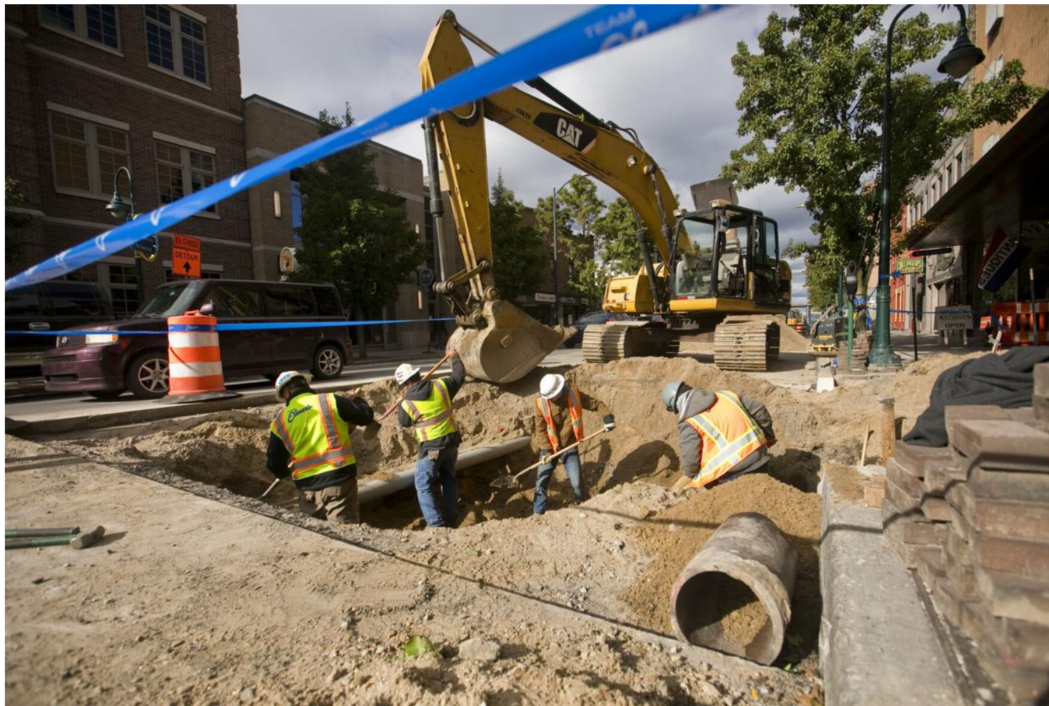
Workers from Team Elmer's dig underneath Union Street for the sanitary sewer, about nine feet down, to work on the line running from Bahia on Tuesday in downtown Traverse City.
