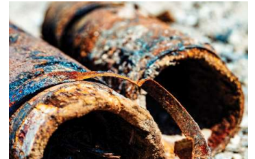
100 yr old steel band wrapped wood water pipe.
